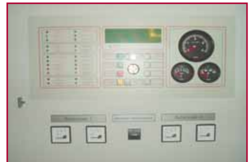
Diesel Pump Controller
