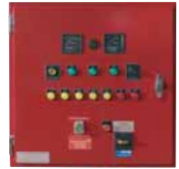
Control panel for jockey pump
