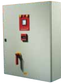
Control panel for the main fire pump
