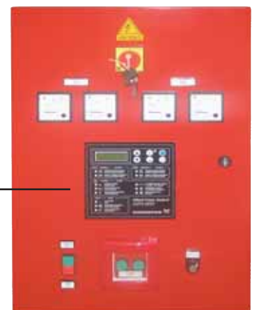
Diesel Pump Controller
