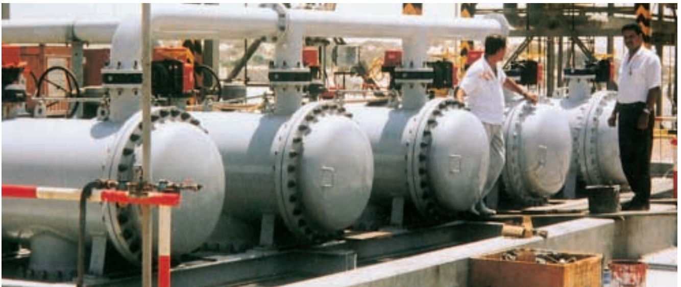
Fig 2. Five Alfa Laval Filters in parallel serve as main inlet cooling water filters for an ammonia plant on the Mediterranean Sea.
