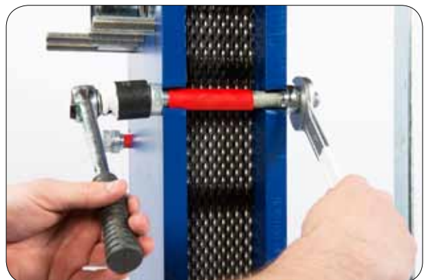
10.5 Tighten the plate heat exchanger to reach the A-measurement that is stated on the drawing of the heat exchanger.
